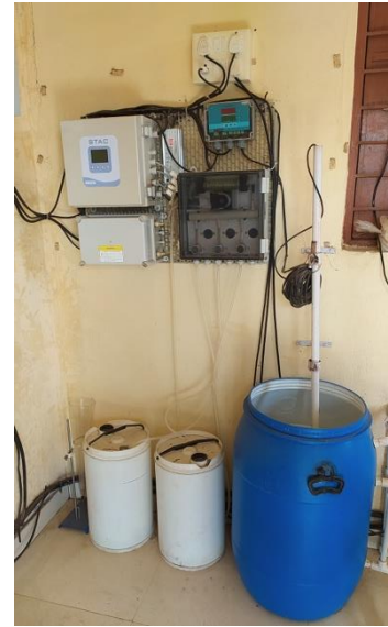
Figure 9 The automated system for monitoring treatment quality in Sinnar
