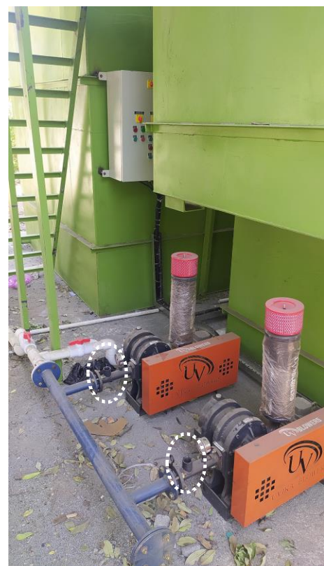
Figure 12 The missing valves of a yet to be commissioned greywater treatment facility located in a park in Sinnar
