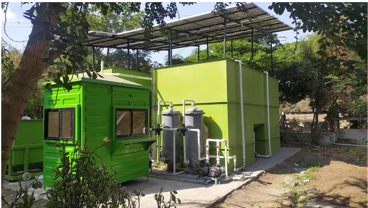
Sinnar is also implementing a decentralised greywater treatment facility located in a park. The 60 KLD moving bed bio-reactor plant is ready for commissioning
